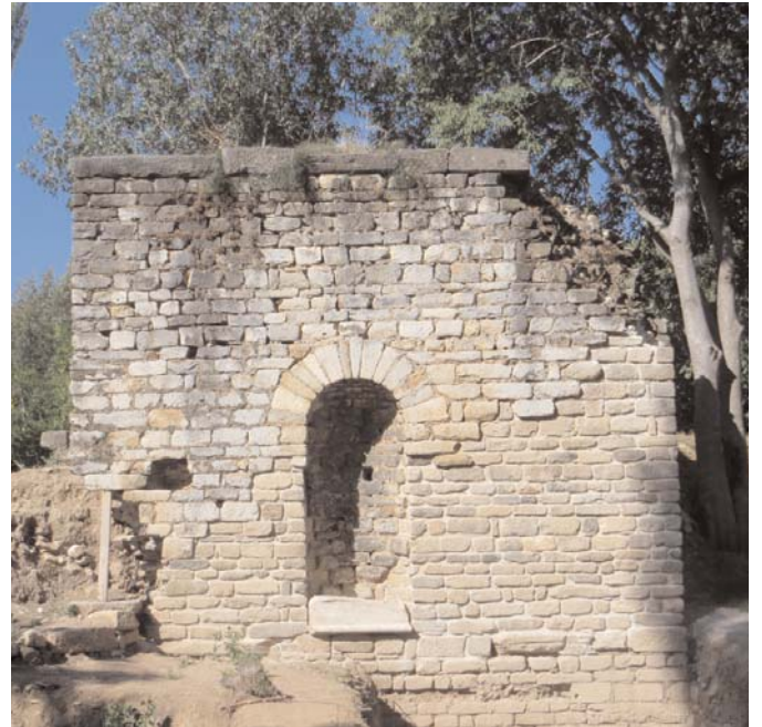
The tall masonry structure on the western side of Tetracylon Street is now repaired and reunited with its inscribed base for Myon Eusebes, found in 2013. A copy of the himation statues – found nearby in 2011 – will be placed on the base next season.
